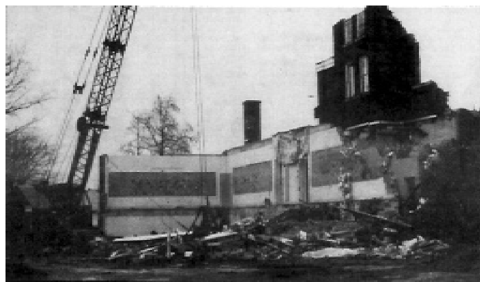
And the walls come tumbling down
